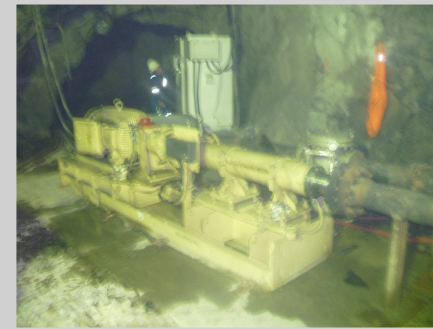
Dewatering - Caverna Mine, Ecuador.
